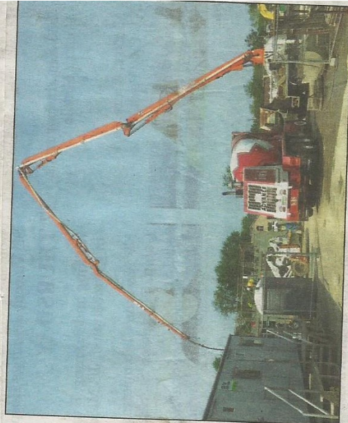
On a rare sunny day earlier this month, crews were able to lay concrete and do other construction work at the city park's new aquatic center. Such days have been rare of late, drastically delaying progress on the $3.2 million project. — Staff Photo by Katy Dudzik
